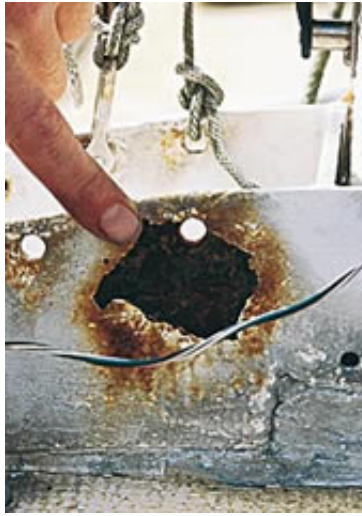
A large rust patch was started by water getting under the protective paint work at the edge of the hole and has resulted in substantial damage.
