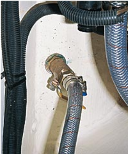
This new bronze skin-fitting (above) is beginning to oxidise. Note the characteristic green colour. The skin-fitting should have been mounted on a block to provide additional strength to the local area of the hull.
